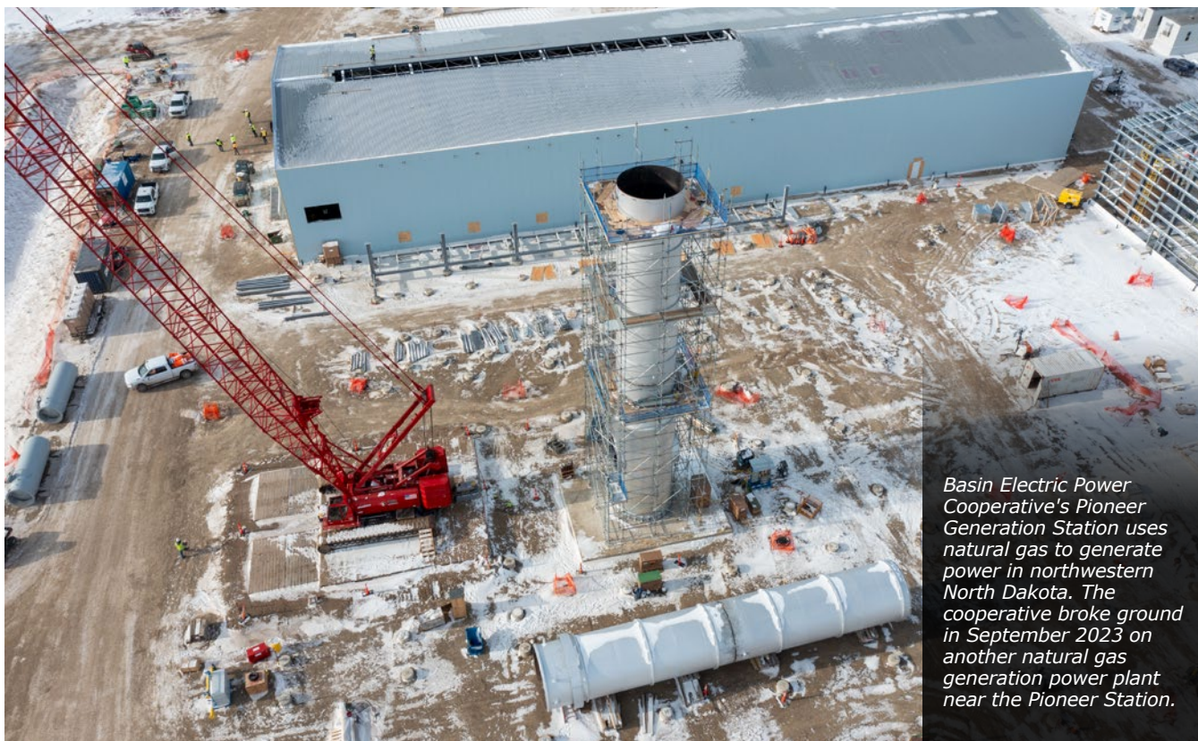
PHOTO COURTESY BASIN ELECTRIC POWER COOPERATIVE
