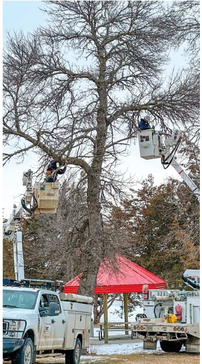
McLean Electric Cooperative lineworkers string solar lights among the tree branches to help brighten area trails.
