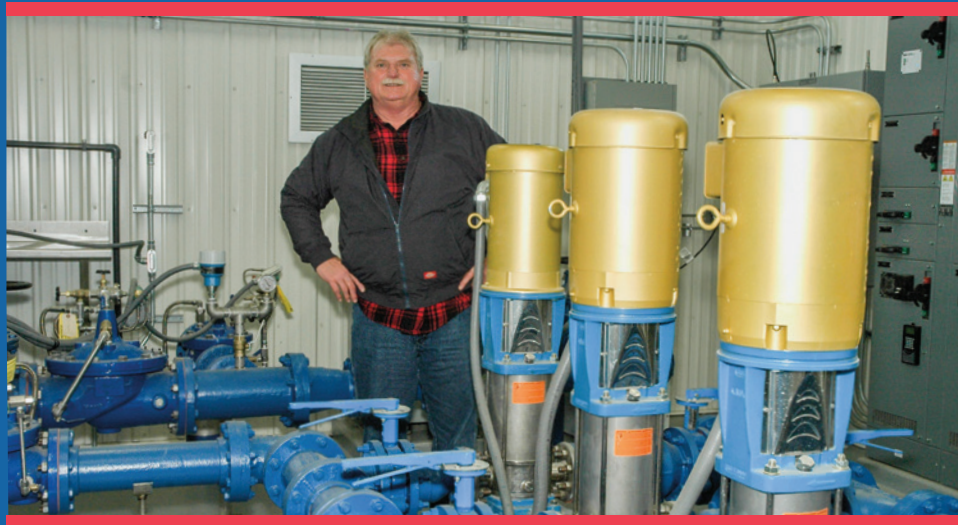
Garrison Rural Water District Manager Todd Martinson in the rural water district’s booster station located east of Garrison. McLean Electric Cooperative serves the district’s two new booster stations and its office.
